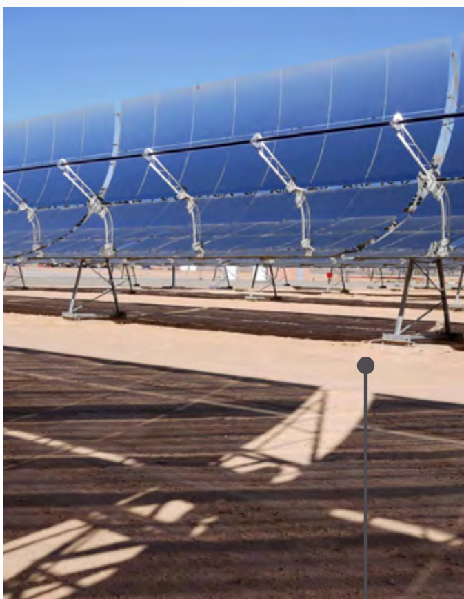
Solar power panels at Ain-Beni-Mathar, Morocco. Photo courtesy Philippe Roos/Flickr
